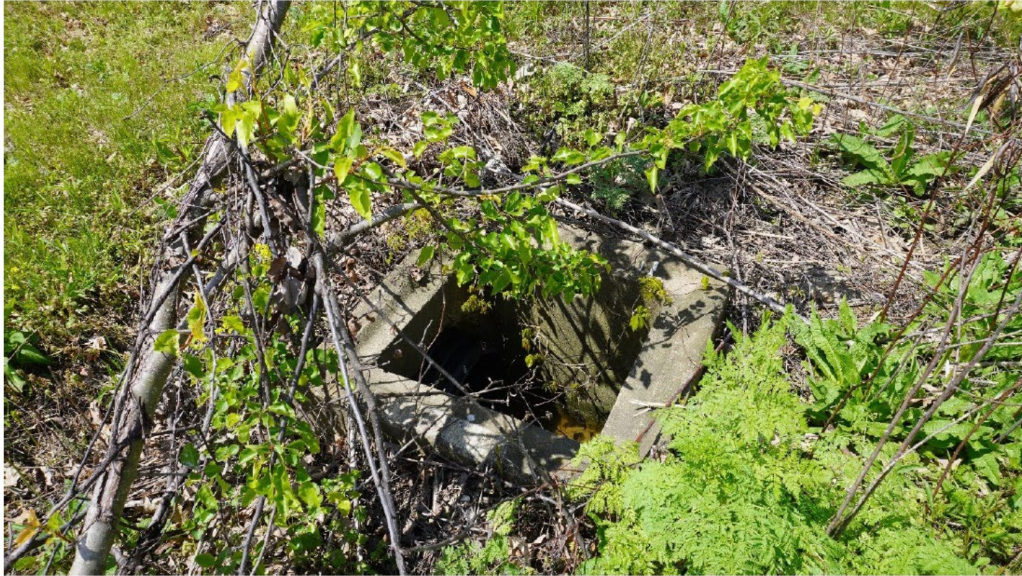
Figure 46: Top view of inlet (with no grate) located NE of the intersection of Professional Park Dr & Business Center Dr (see above)
