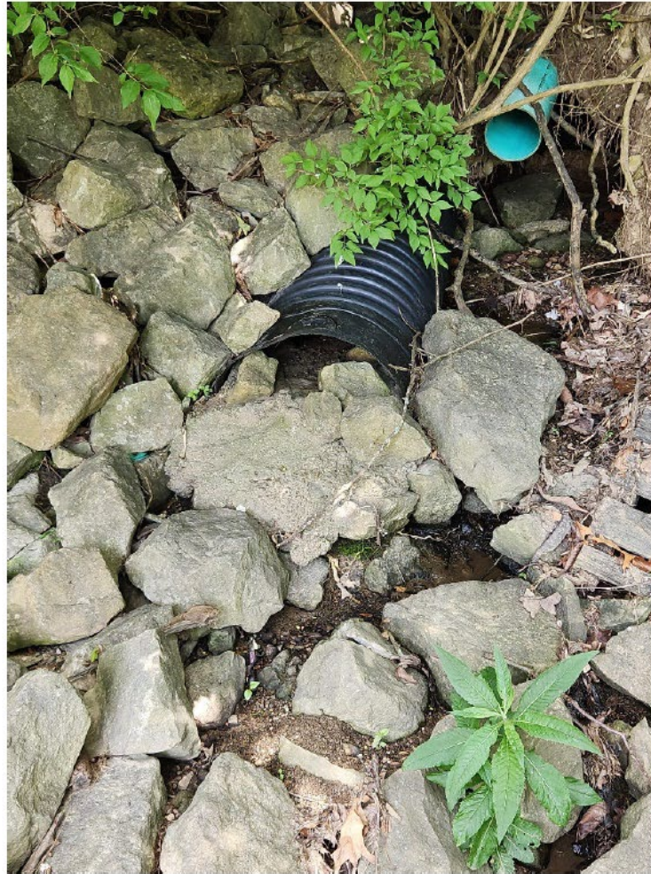
Figure 69: Obstructed stormwater outlet behind existing St. E's MOB & gutter outlet (running east to west, size unknown)
