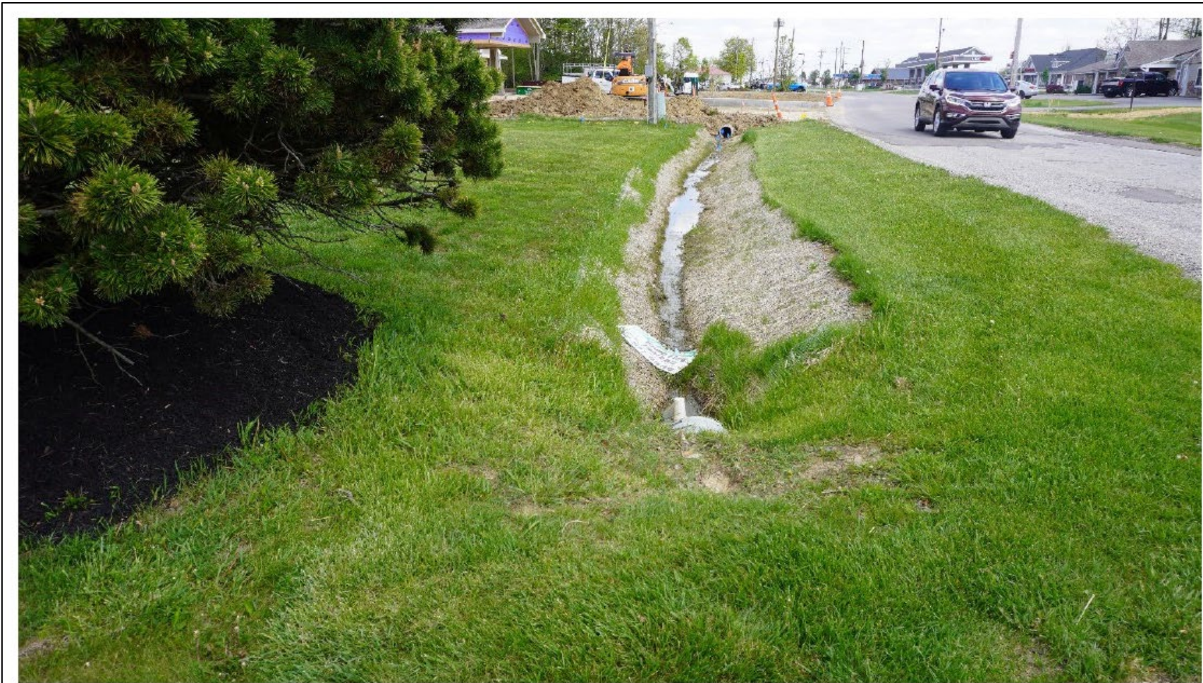
Figure 60: Drainage ditch along Jamison Dr just east of Professional Park Dr (looking east)
