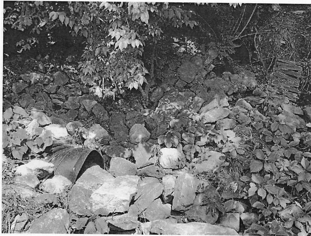
Figure 70: Two obstructed stormwater outlets behind existing St. E's MOB & gutter outlet
